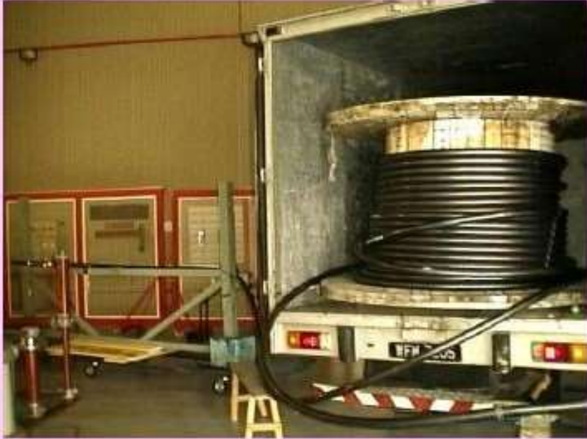
High voltage AC withstand test on 11 kV XLPE single core cable (TOPLINK SDN BHD)
